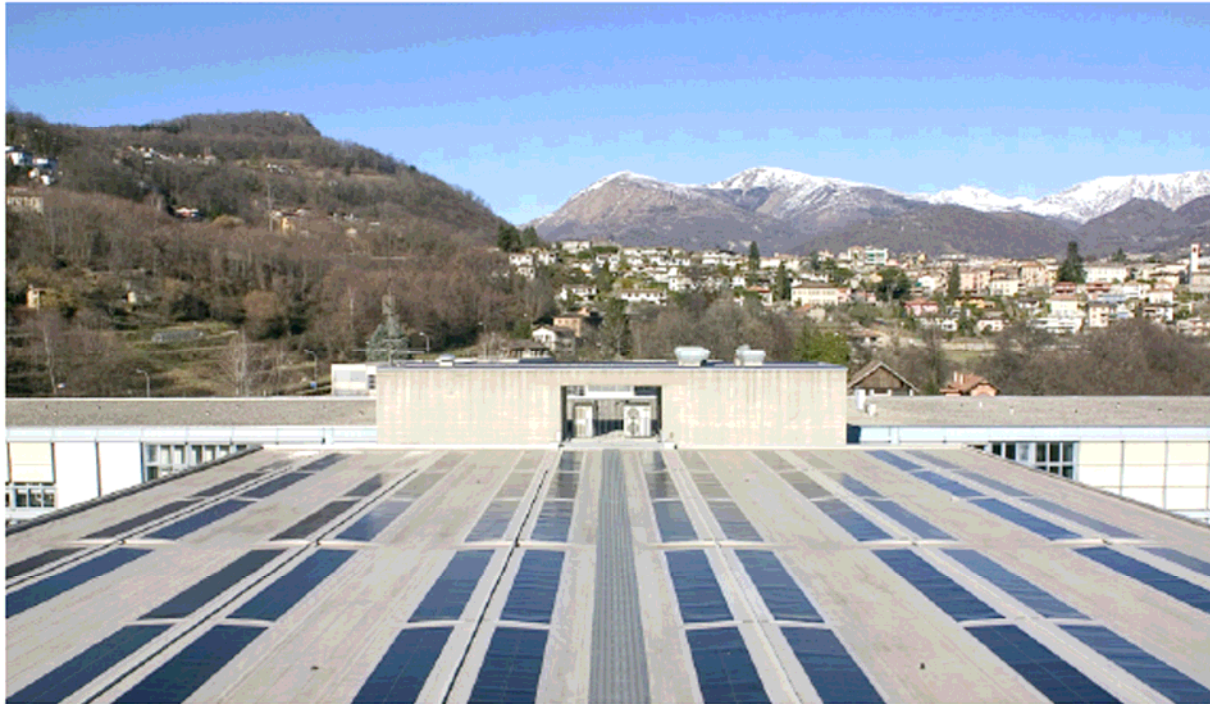
Fig. 1. Thin film PV modules laminated together with polyolefin membranes which act as a waterproofing system.
